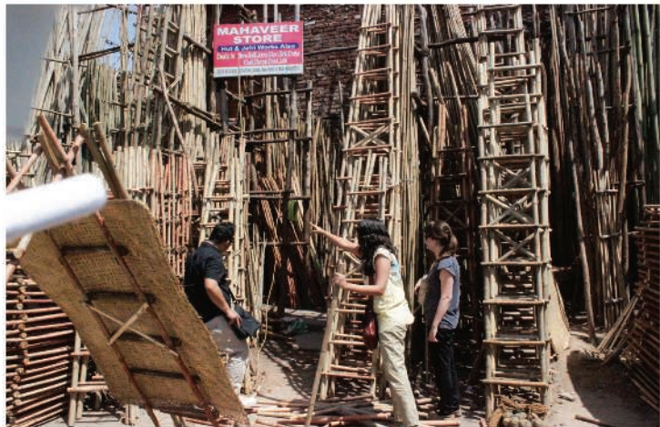
Made up of locally available and affordable materials such as bamboo, rebars and waterproof canvas, the shelter also uses the simple local skills of a welder to make the joints and a tailor to stitch the skin (above).
